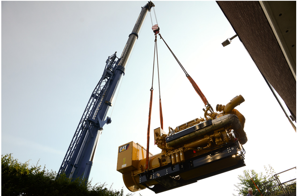
Delivery of the new CHP generators in 2013
